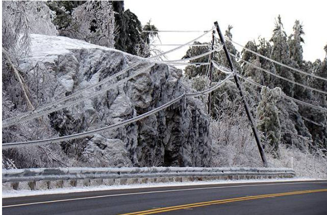
The aftermath of the 2008 ice storm
